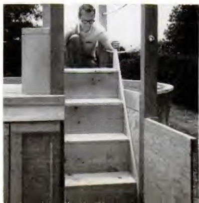
HOMEOWNER-BUILDER lowers prebuilt stairs into position. There's space at bottom for small footbath
